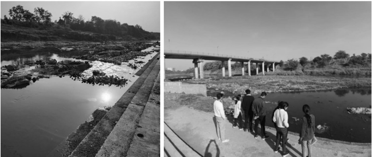
Figure 12. Confluence zone showing concretization, algae, hyacinth formation (left) water getting clogged due perpendicular bridge. (right)
