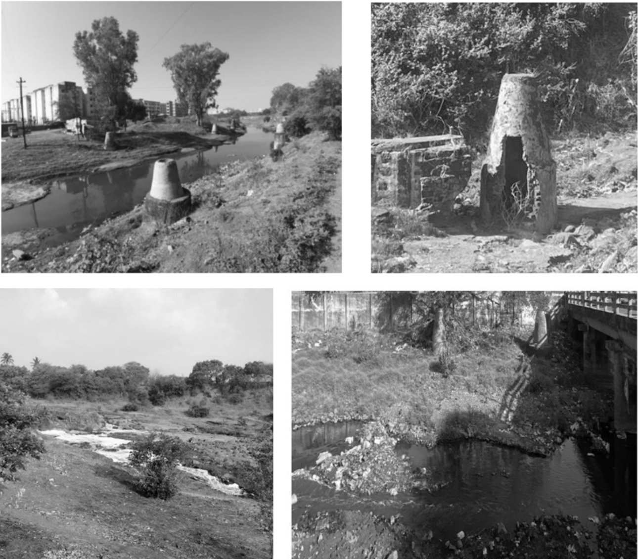
Figure 13. Various issues like sewers running along river banks (top left), broken sewers (top right), foam formation (bottom left) and solid waste thrown in Nandini (bottom right)
