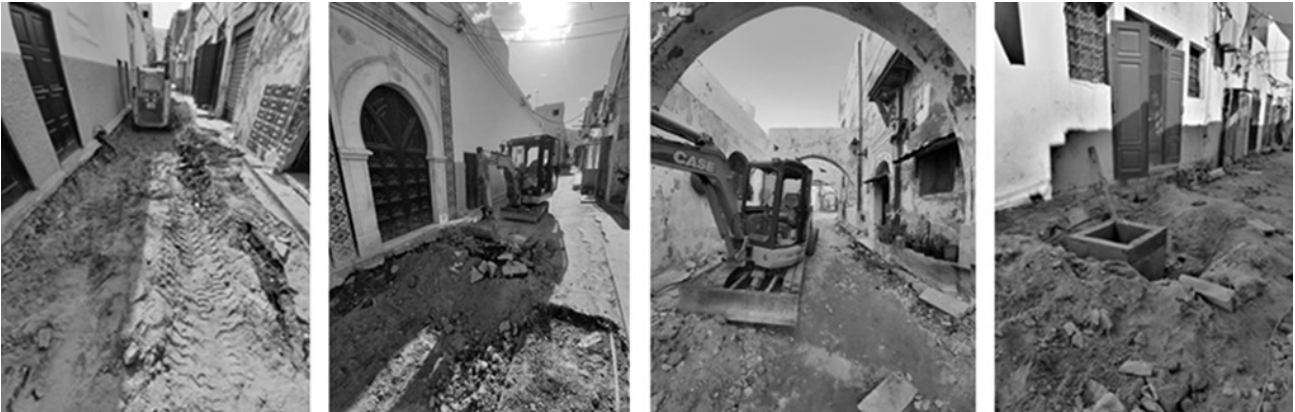
Figure 15. Bulldozers were used to remove the historic street pavement of Tripoli's old city and dig the ground for water and sewage system maintenance. Source: OCTAB's Facebook page (Accessed August 2023).
