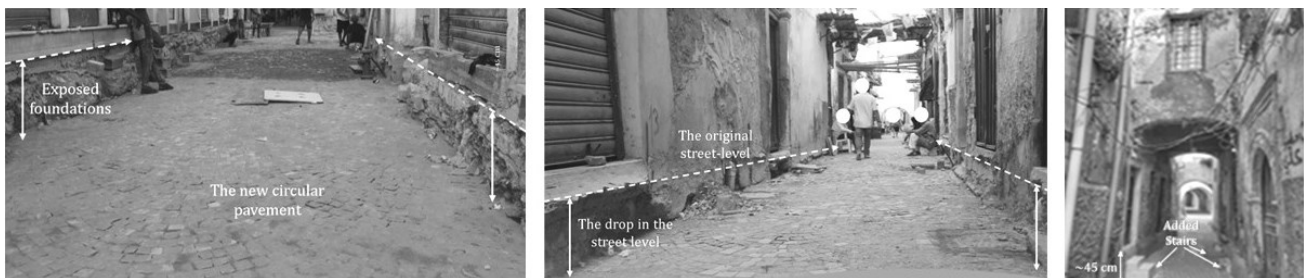
Figure 18. The differences in street elevation and buildings' doors created due to a lack of informed street paving practices. Source of left two images: OCTAB Facebook page (Accessed September 2021). Source of right image: Zawaia Trablusia Facebook page (Accessed May 2024).
