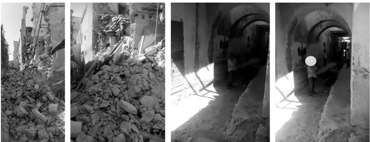
Figure 16. The collapsed building on Kosha Al Soffar Street in Tripoli's old city. The collapse was due to excavation works. Source: Facebook pages: Save the Old City and Tik (Accessed July 2023).
