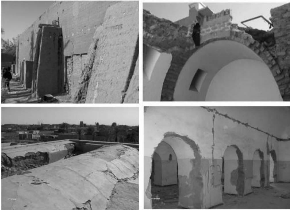
Figure 3: Deteriorated parts of the historical hospital of Adrar
